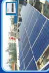
SOLAR POWER PLANT
