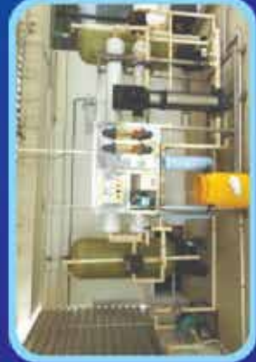
AUTOMATIC INDUSTRIAL RO
